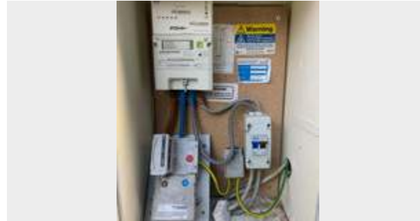
Your main electricity supply - this must be a clear photo showing the cabling running into the supply
