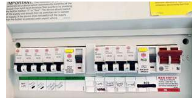
Your main fuse board and any others you have – we need to be able to see the board up close with clear labels and breakers
