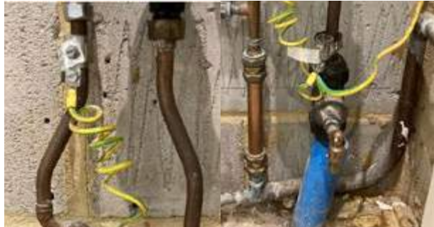
The protective mains bonding arrangements supplying your home such as oil, gas, and water
